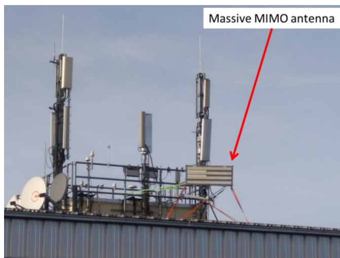
Figure 2.25: Massive MIMO antenna of 64 antenna elements (4 lines and 16 columns of antenna elements) on the roof of a building of Nokia Bell Labs campus in Stuttgart.
